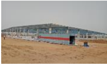
Our new plant under construction in Rajasthan State (Planned to start mass production in 2019)
