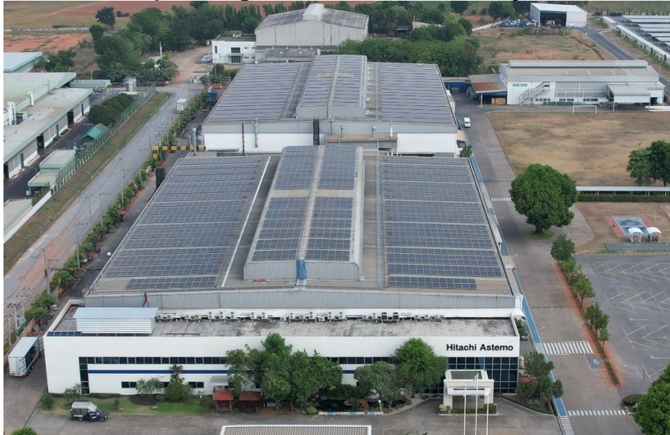
Solar panels on the roof of Korat Plant #3
